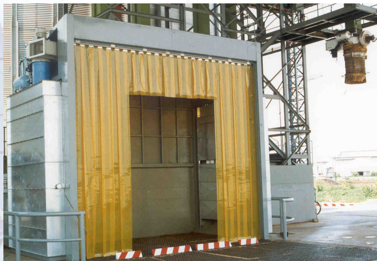
Thailand, Vegetable Oil Plant 2 x JM 20/25 20,000 Am 3 /h
