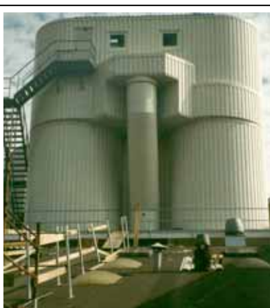
Boiler, Coal 3C Twin Module
